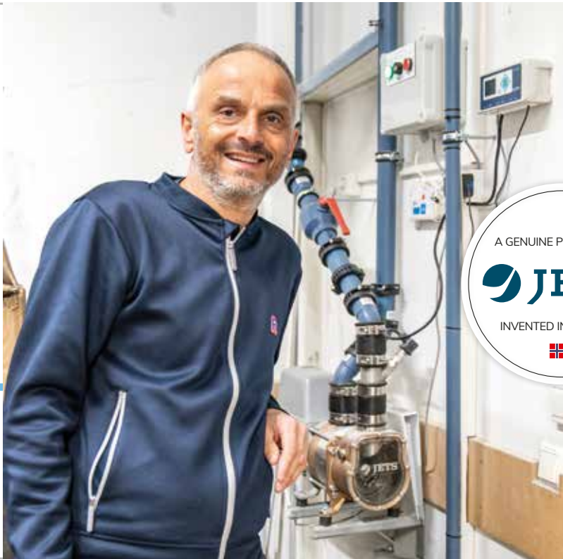
A single Vacuumarator® pump serves the entire vacuum drainage system at the REMA 1000 store in Ulsteinvik, Norway.
